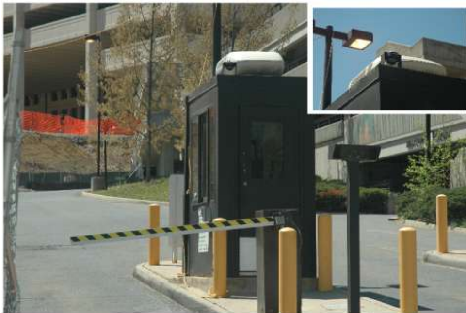
Figure 3.2: Image of Camera Installation
